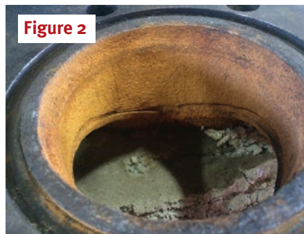
Sand dropout and internal weld corrosion inside a welded pipe manifold
